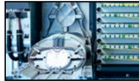
Optical Distribution Frames
